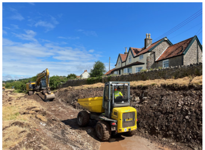
Creating a new cutting between Erlon Lane and the A371 at Easton.
