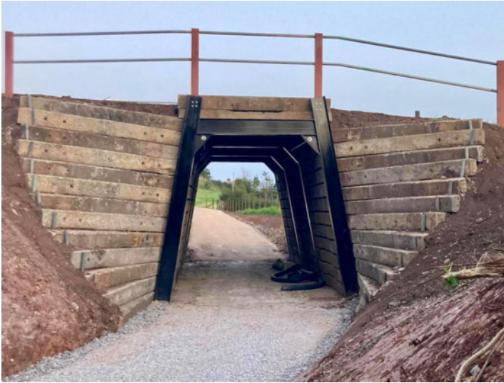
A stunning new farm accommodation bridge, designed by John Grimshaw and constructed by MP & KM Golding, has been put in place at Easton.
